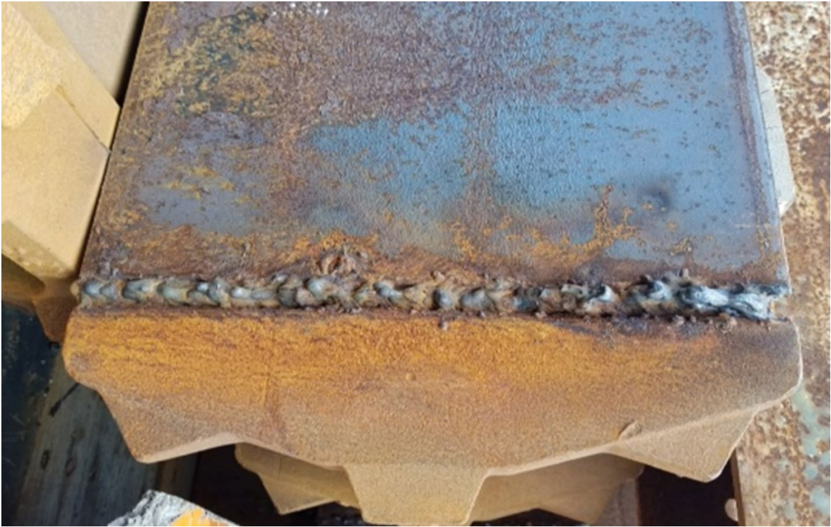
Underfilled joint, lack of fusion, unacceptable profile
