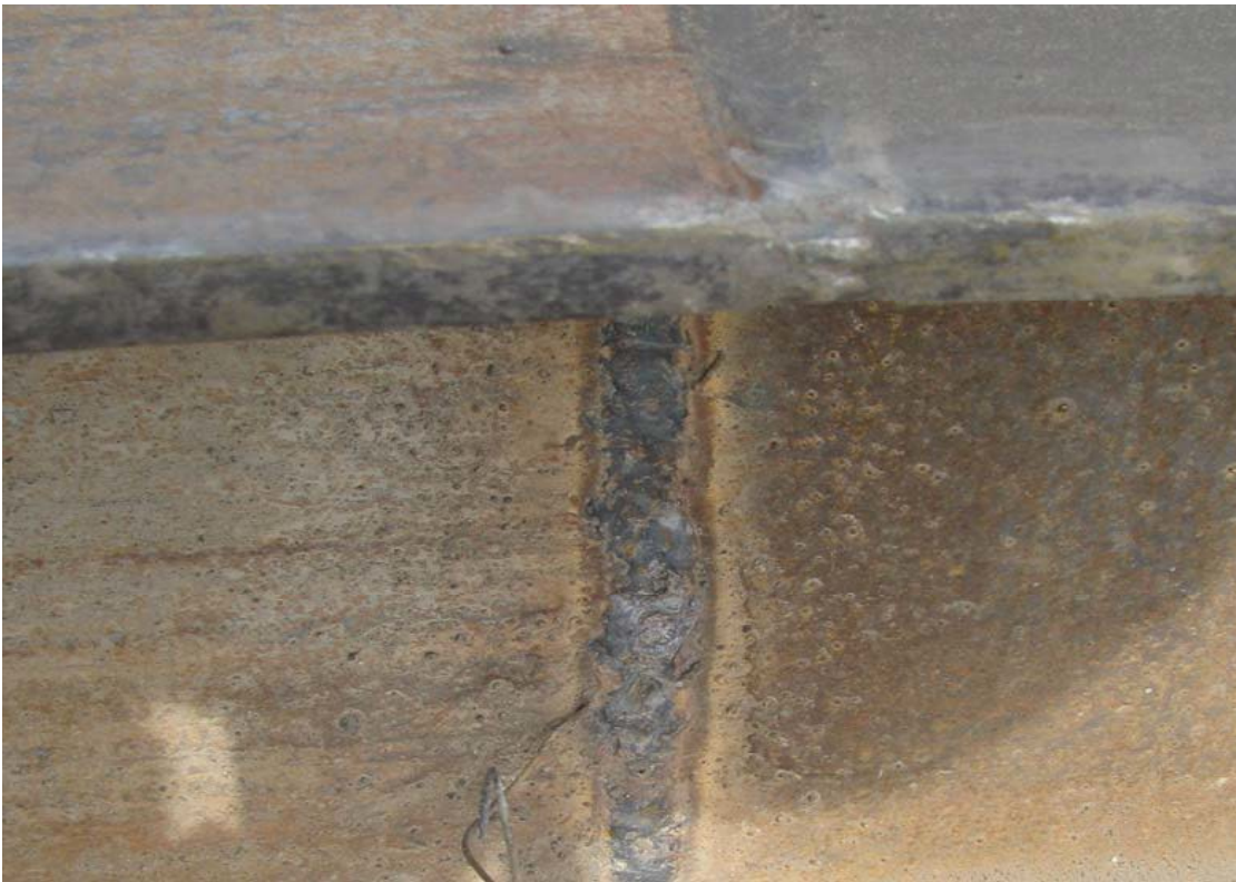
Under fill, use of an unapproved wire fed process (GMAW) - note wire protruding from weld.
